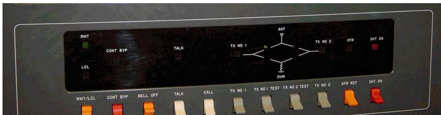
Close up of control panel
